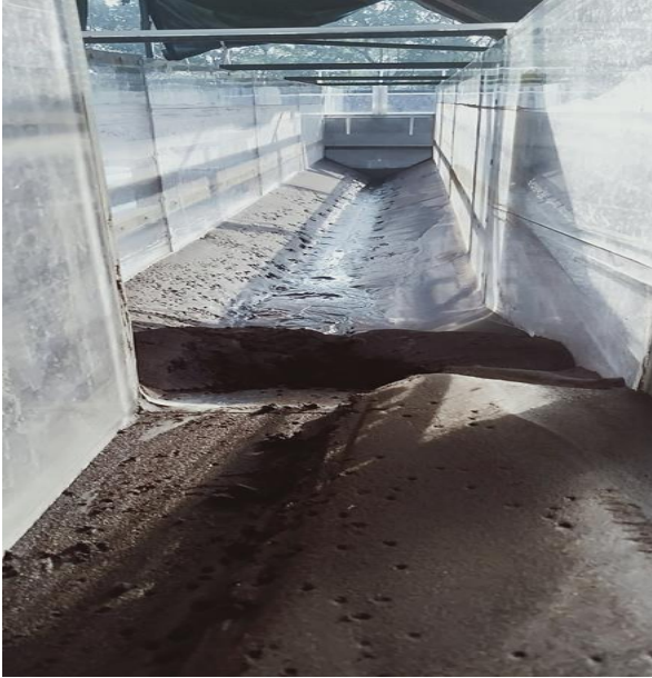
Photograph 1. Typical pattern of deposition inside the desander basin
