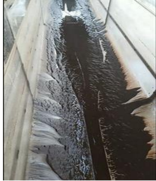
Photograph 2. Drawdown flushing under progress (desander basin)
